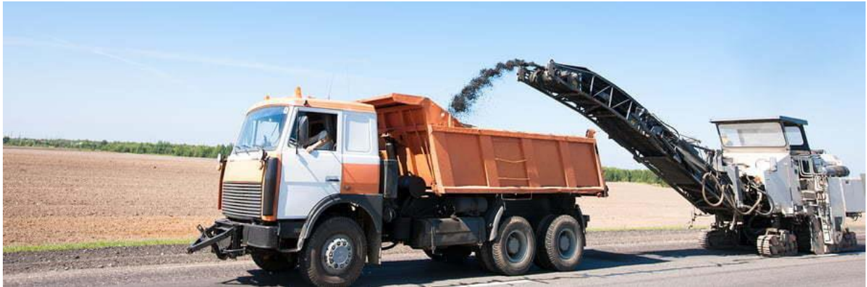
Milling machine loading crushing asphalt into dump truck during repairing road works
